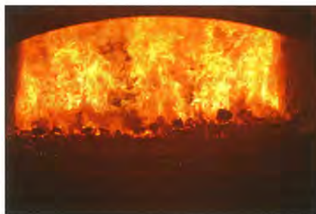
Blick in die Brennkammer
