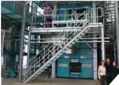
Image detailing a 7.8 MWth CHP plant in the Netherlands
