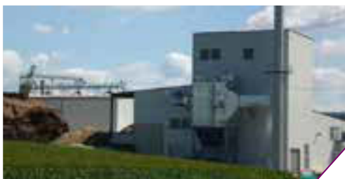
Image detailing the fuel yard, the sawdust dryer and the CHP plant
