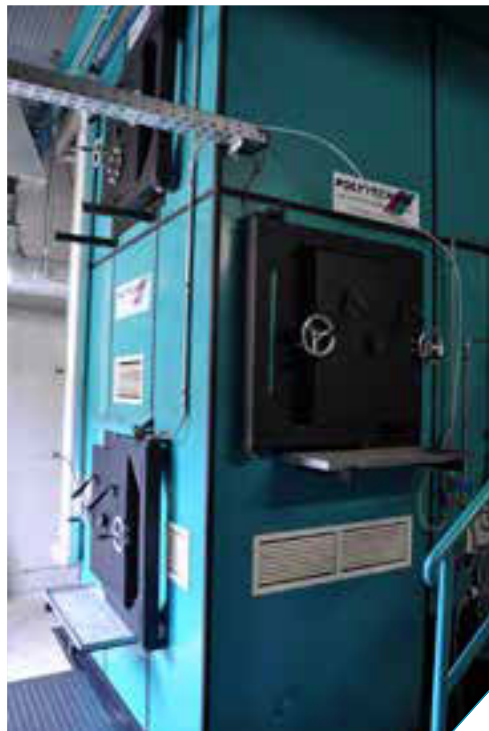
Image detailing the 1 MW R&D plant
