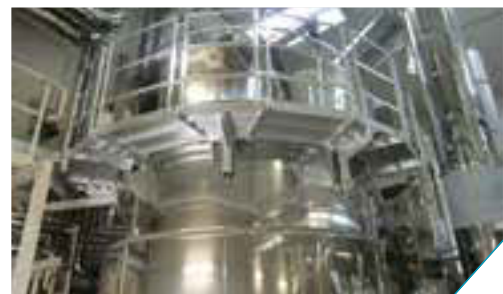
Image detailing the thermal oil heat exchanger of an ORC CHP plant
